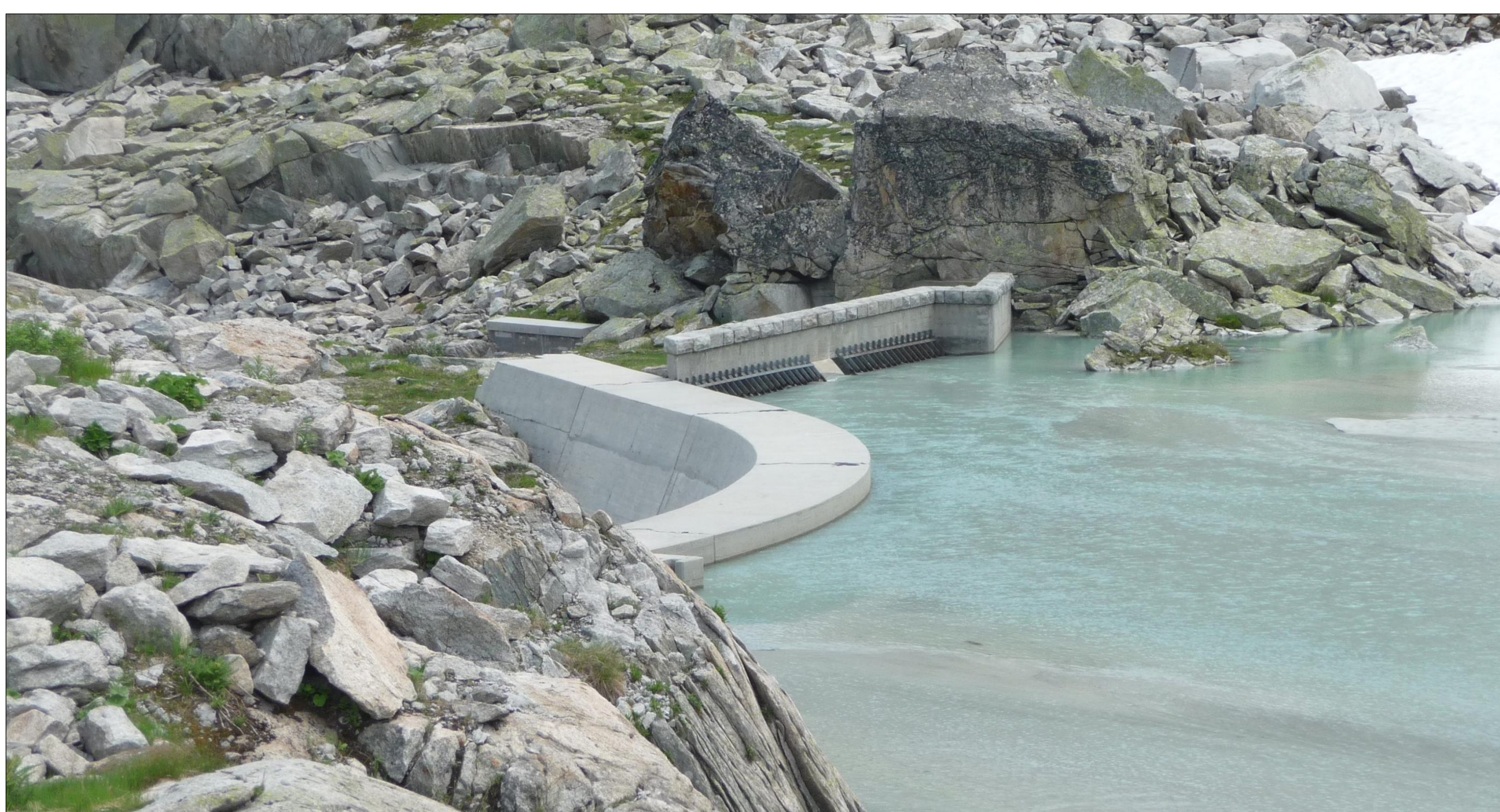
Figure 2. The Bächlibach dam which diverts the water into the Bächli gallery. The water intake is equipped with a trashrack to avoid big stones to enter the gallery. The capacity of the water intake is 7.5 m 3 /s.
