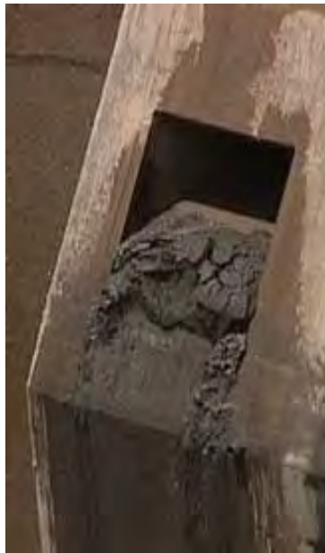
Bottom outlet partially blocked by sediments at the Jiroft Dam, Iran (Photo by S. Emami)
