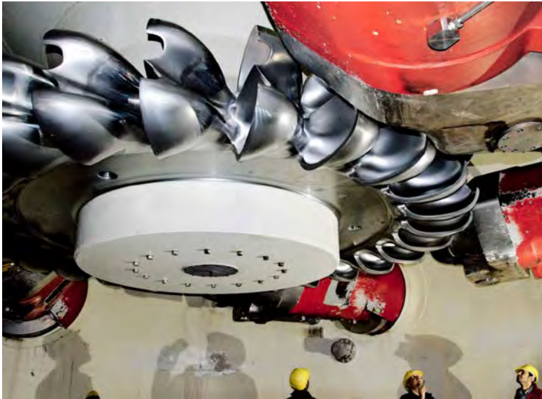
Bieudron Pelton Turbine
